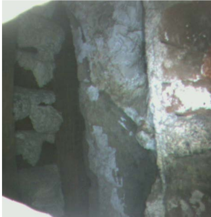
Figure 5: View from scope showing both masonry back-up (to right) and plaster and lathe back-up (to left).
