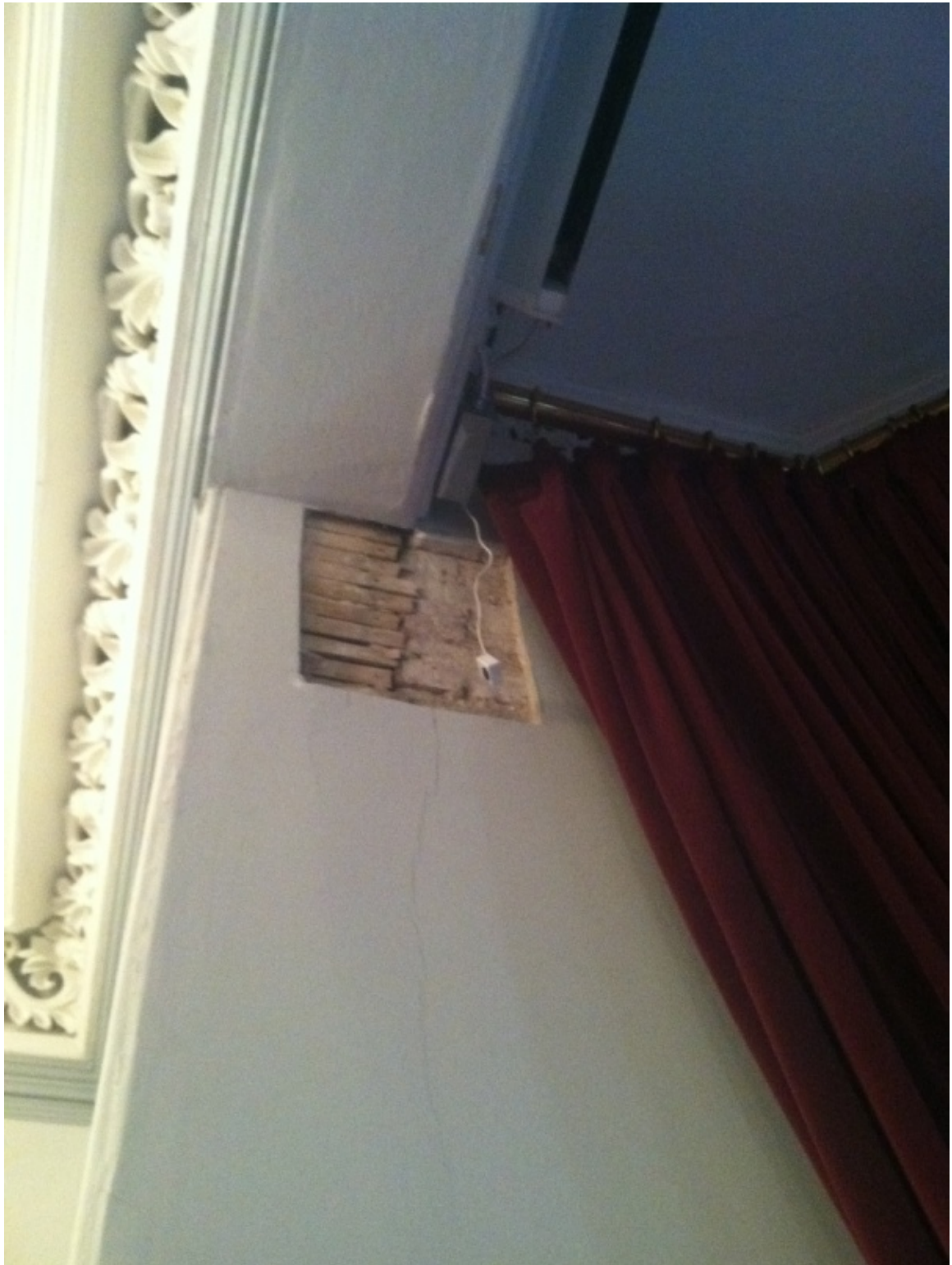
Figure 4: Probe location at eastern side of bay window opening in Regent's Room.
